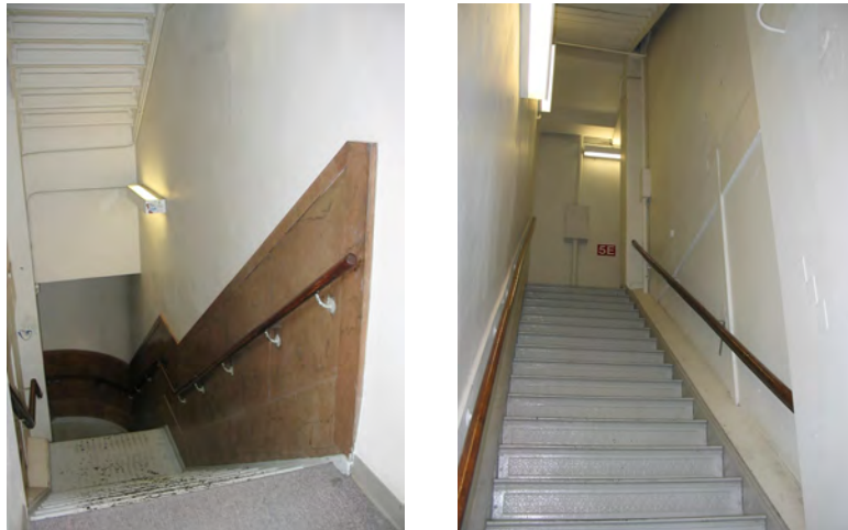
East Stairway looking down from the second floor (left) and looking up at typical flight (right)
