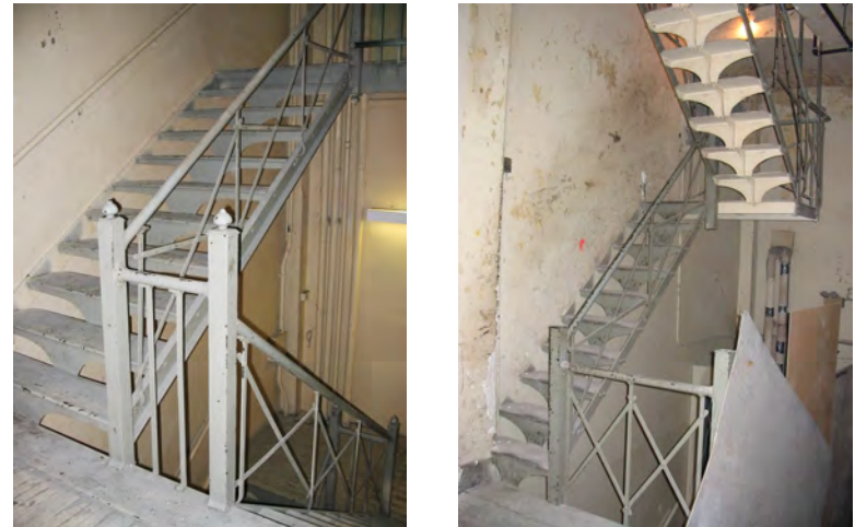
West Stairway, typical configuration (left) and view of the more narrow stairs up to the roof (right)
