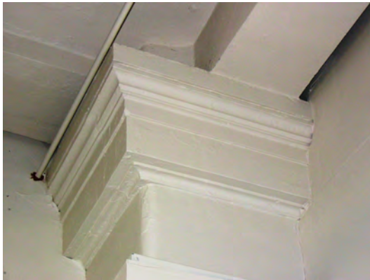
Detail of plaster pier capitals that can be found throughout the building
