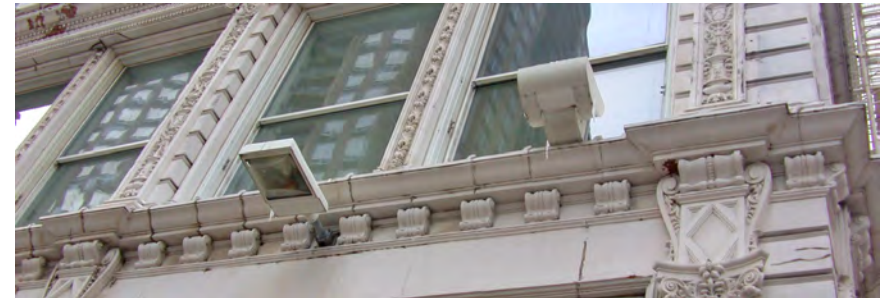
Exterior elevation – HID floodlights mounted to building façade.
