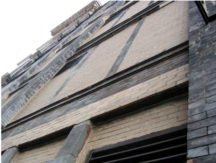
View of bricked-in window openings and existing terra cotta trim and mullions at upper floors of West (alley) façade
